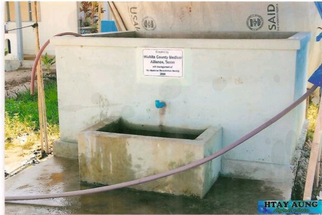
One of the 5 tube wells/water pump and container that was sponsored by the Wichita County Medical Alliance.
